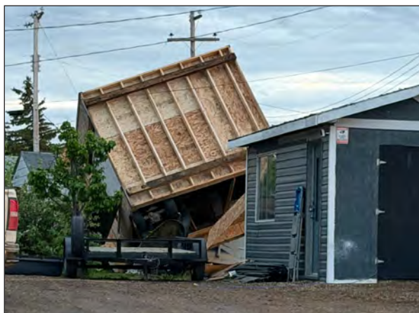
In Girouxville on Monday a fair amount of damage was done, including some homes may have to be written off.
